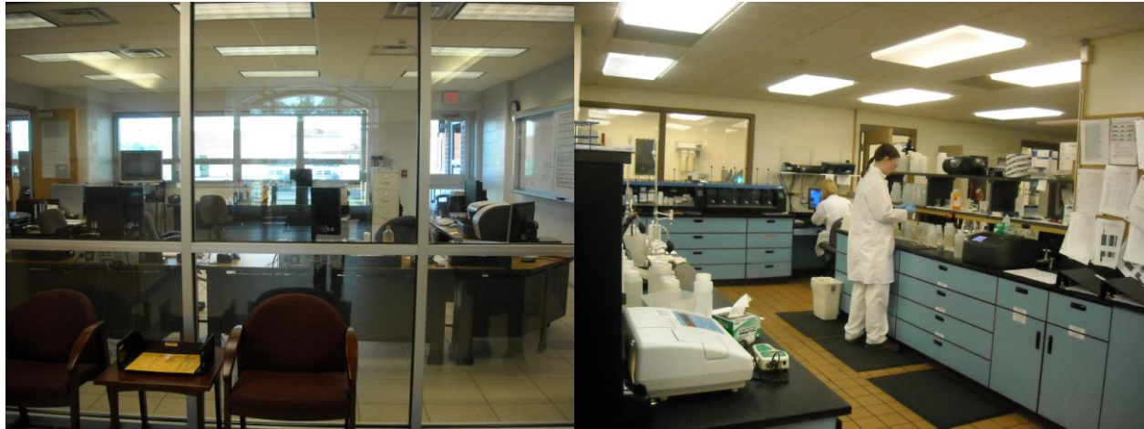
Northwest River Water Treatment Plant – Control Room and Laboratory
