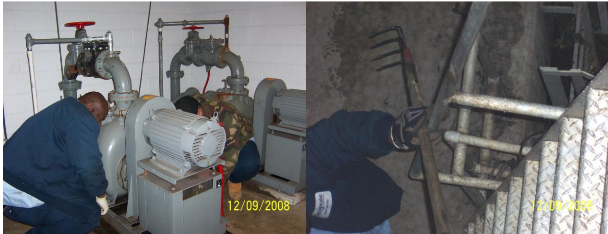
M&O – Sewer finishing maintenance on a pump and removing waste from a grate
