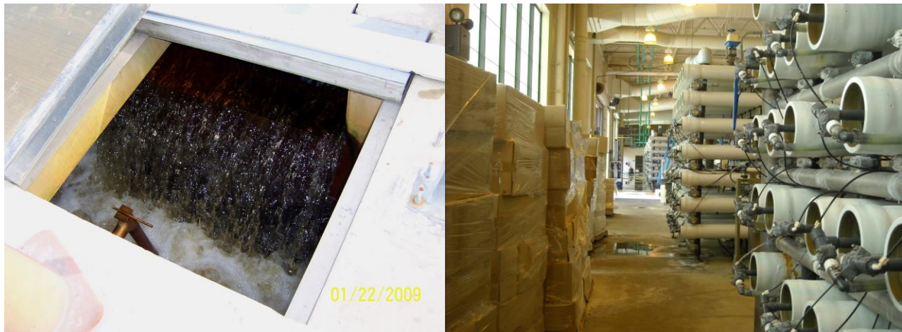
Lake Gaston Water Treatment Plant – Early Stage Processing and Micro-fiber Filtration System
