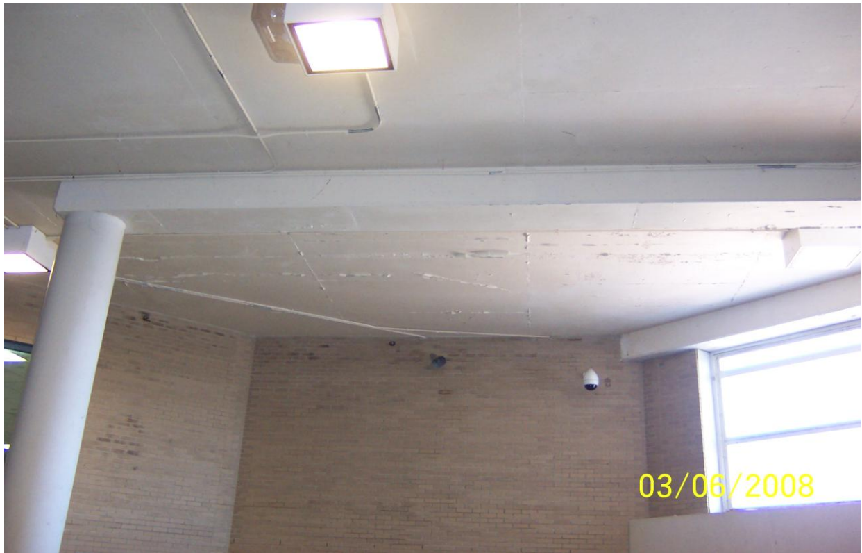
Flaking and Peeling Ceiling Paint
