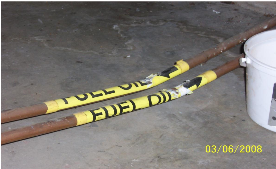
Bent Diesel Fuel Line
