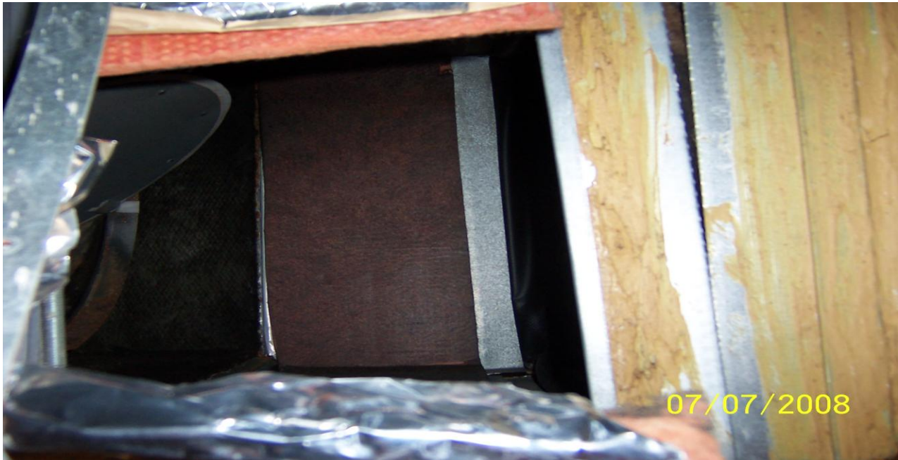
Missing Variable Air Volume box from open day area – Pod 2C
