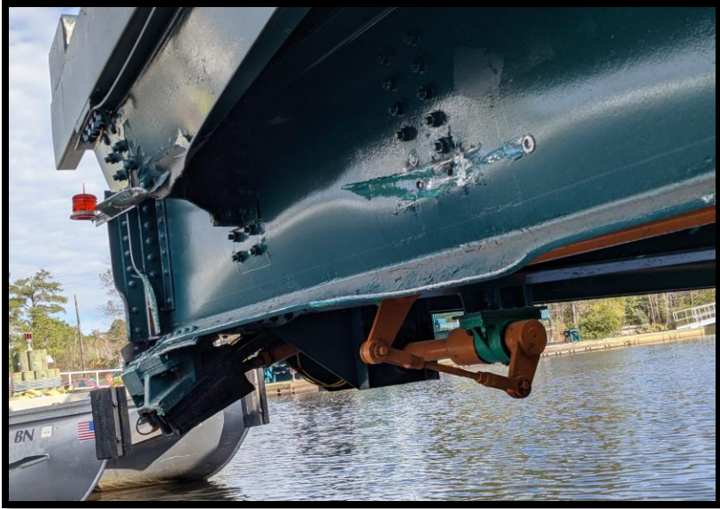
Floor Beam Damage (Fracture Critical Member)
