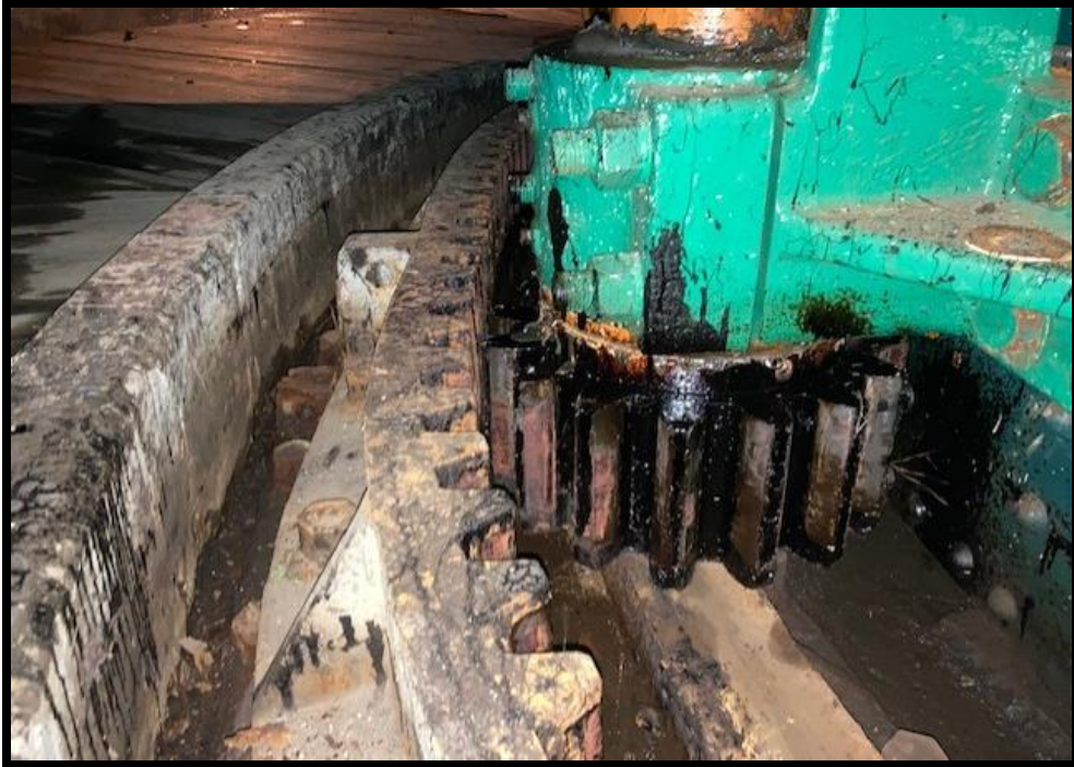
Drive Gear Misalignment / Damage to Rack / Track
