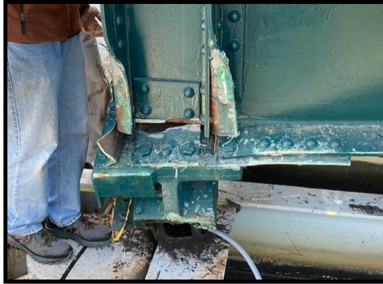
Gusset Plate Damage (Fracture Critical Member)
