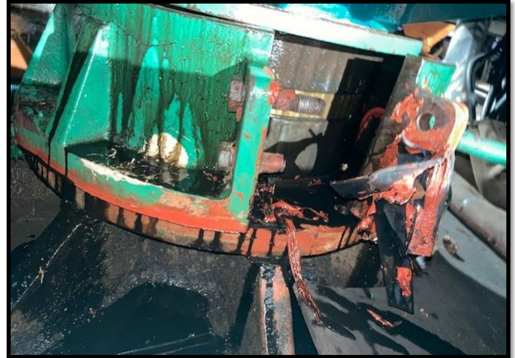
Pivot Bearing Housing Damage
