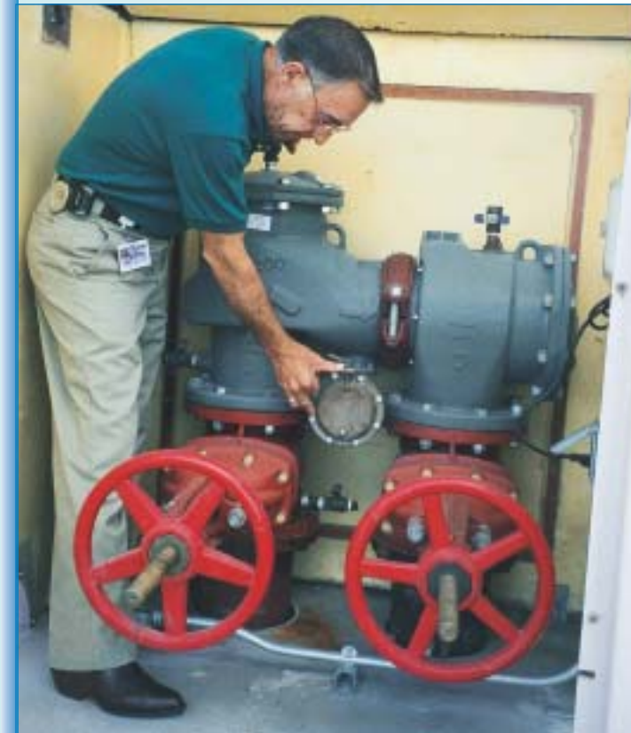
Cross connection inspector examines industrial back flow device
