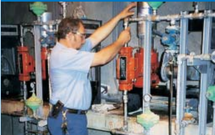
Water plant maintenance mechanic checking chemical feed system
